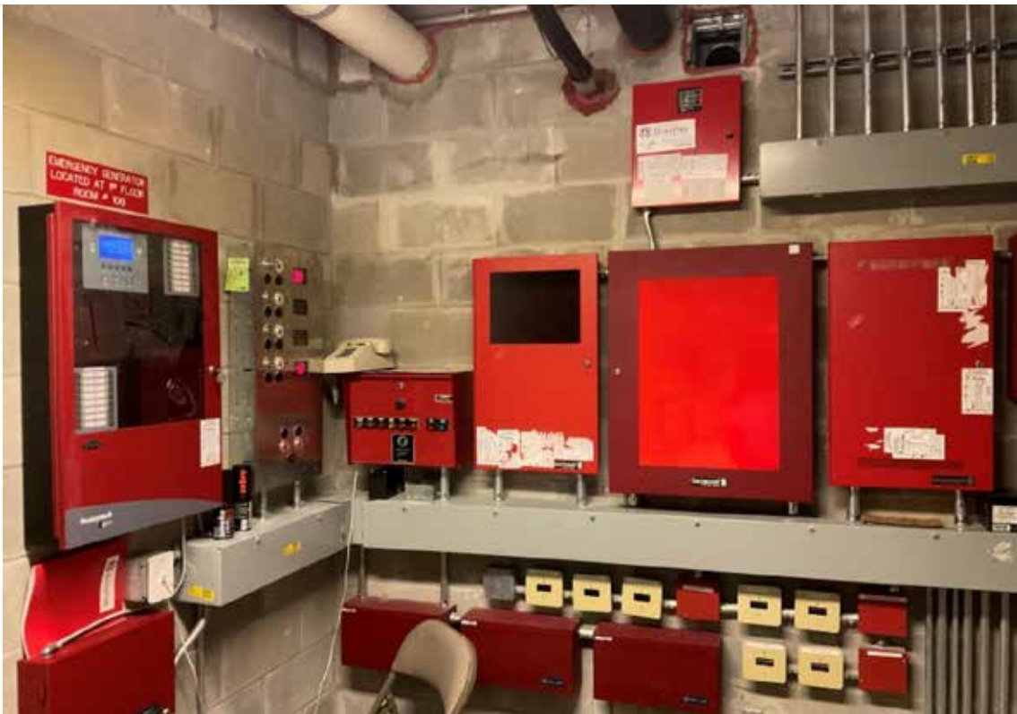
Fire Alarm Control Panel
