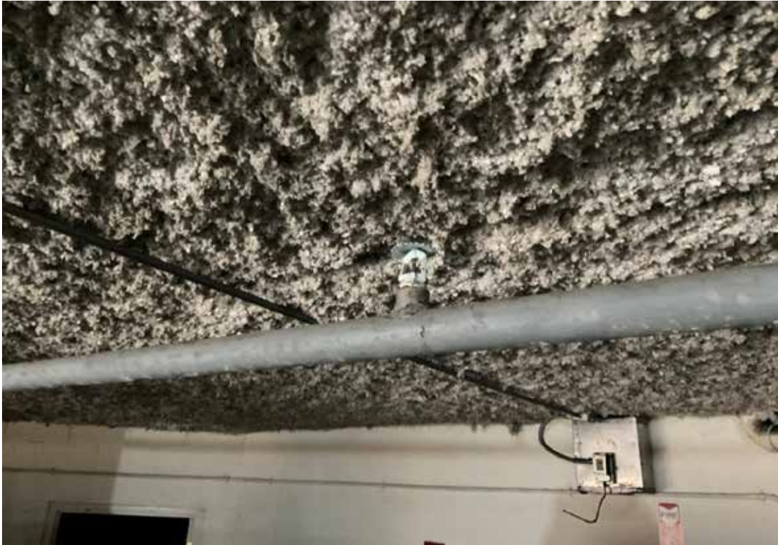
Fire Sprinkler Head
