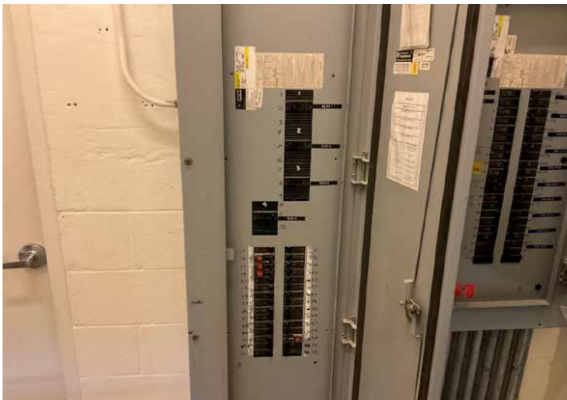
Electrical Panel REM
