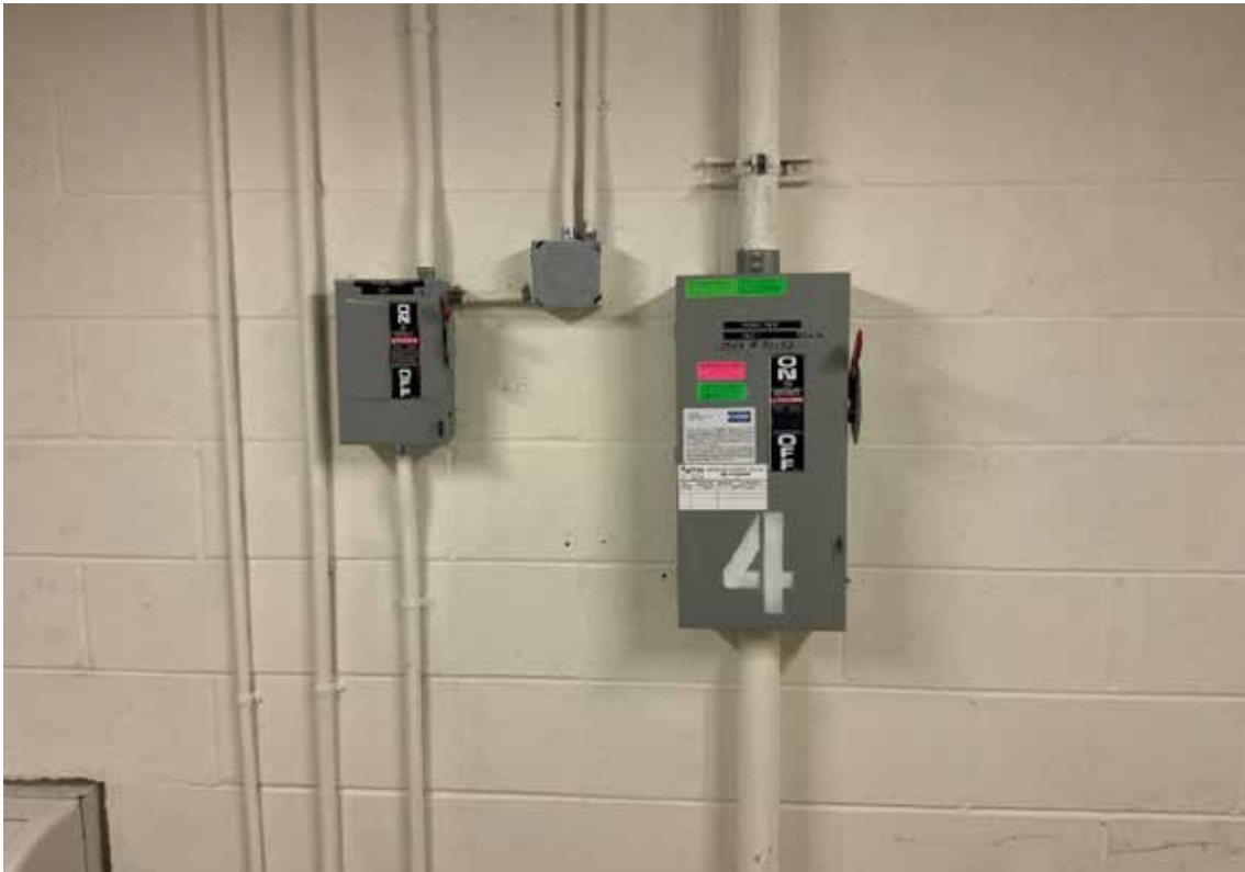
Elevator Control Shut Off
