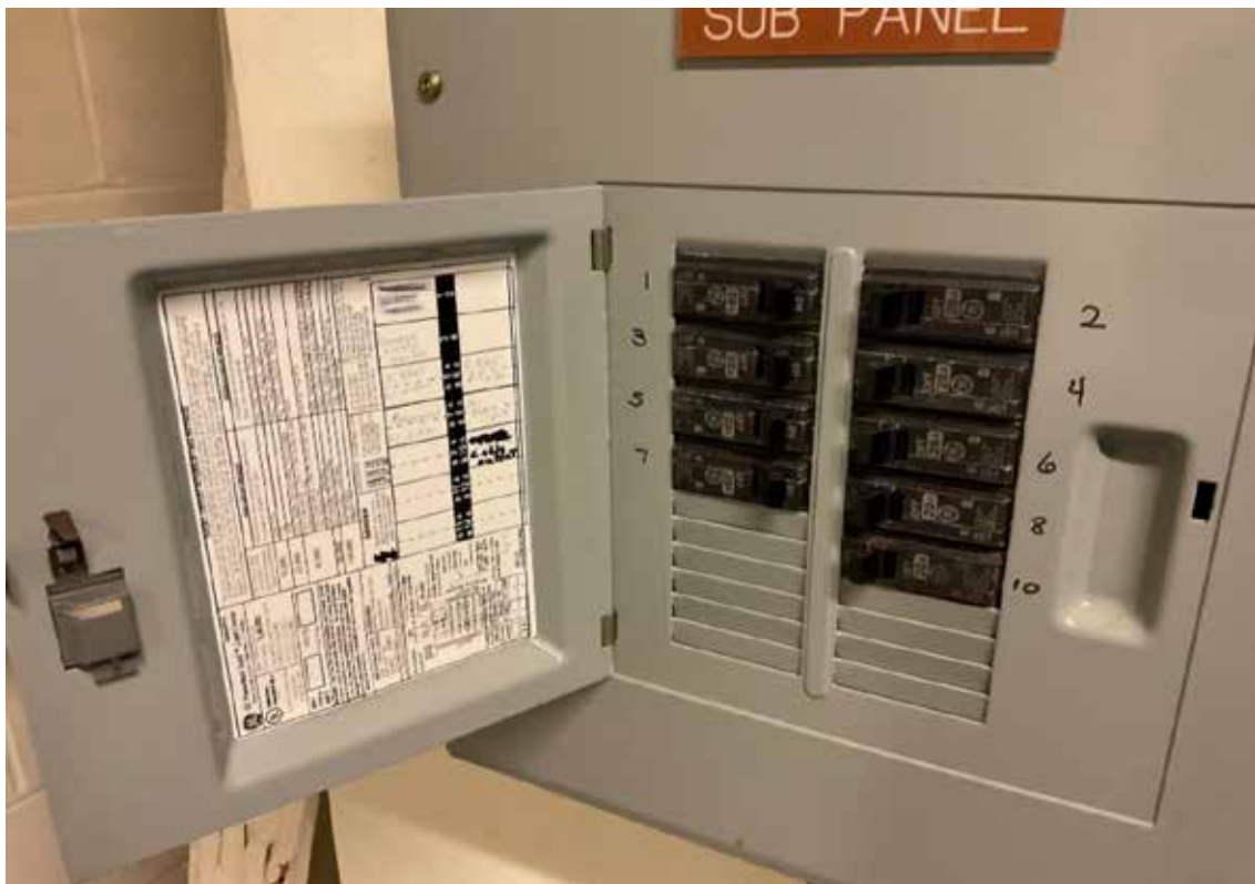
Electrical Panel 1EM Sub
