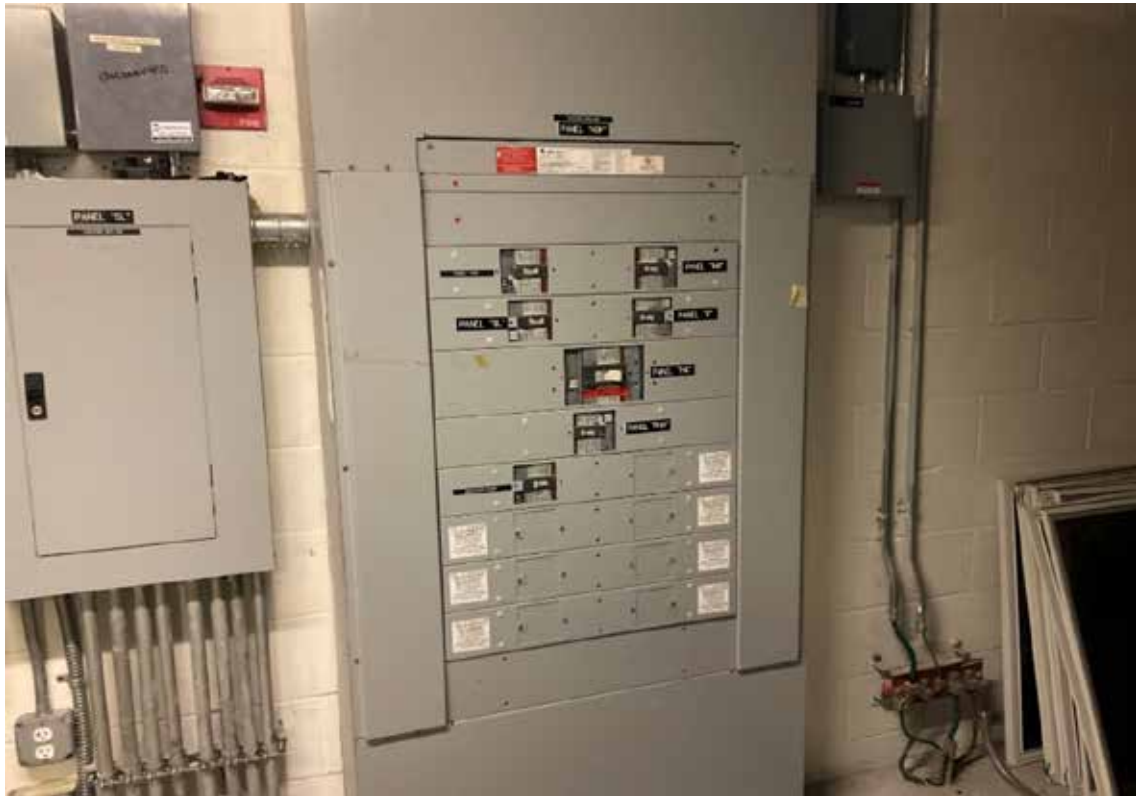
Electrical Panel HDP
