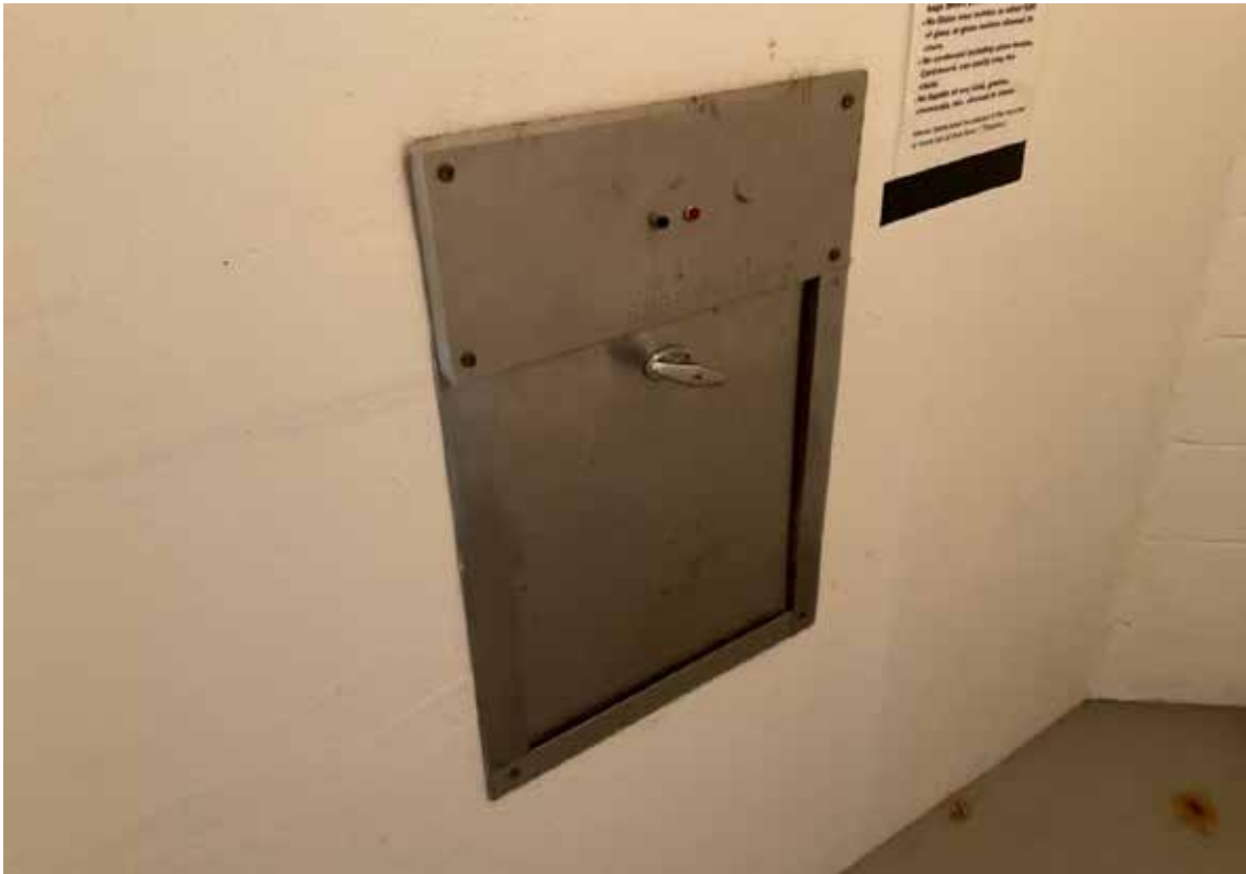
Trash Chute Intake
