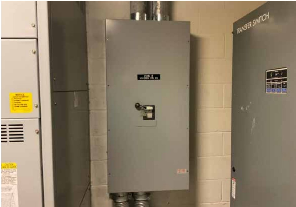
Electrical Panel ECBB
