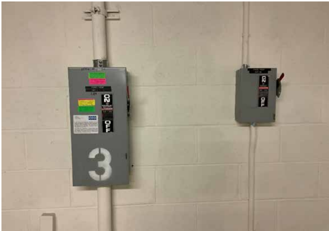
Elevator Control Shut Off
