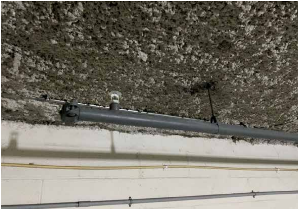
Fire Sprinkler Head
