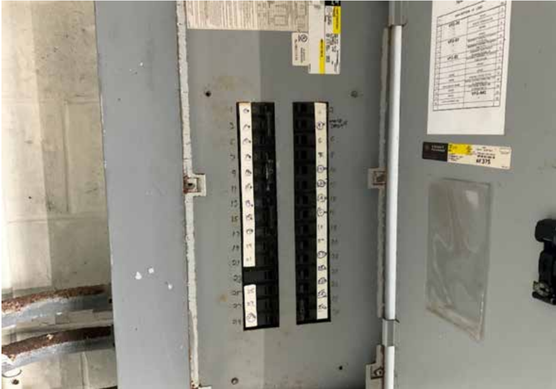
Electrical Panel 1HA
