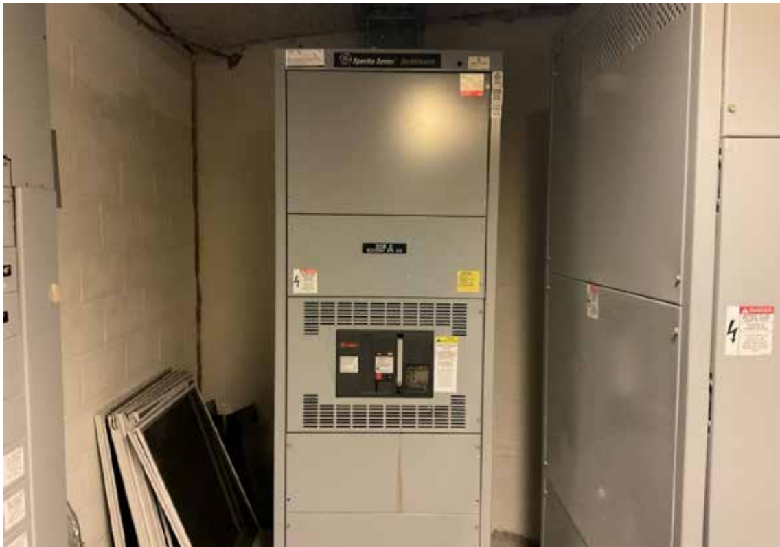
Electrical Panel ECBD
