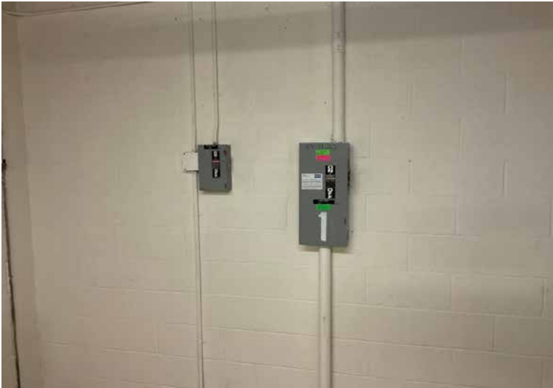
Elevator Control Shut Off
