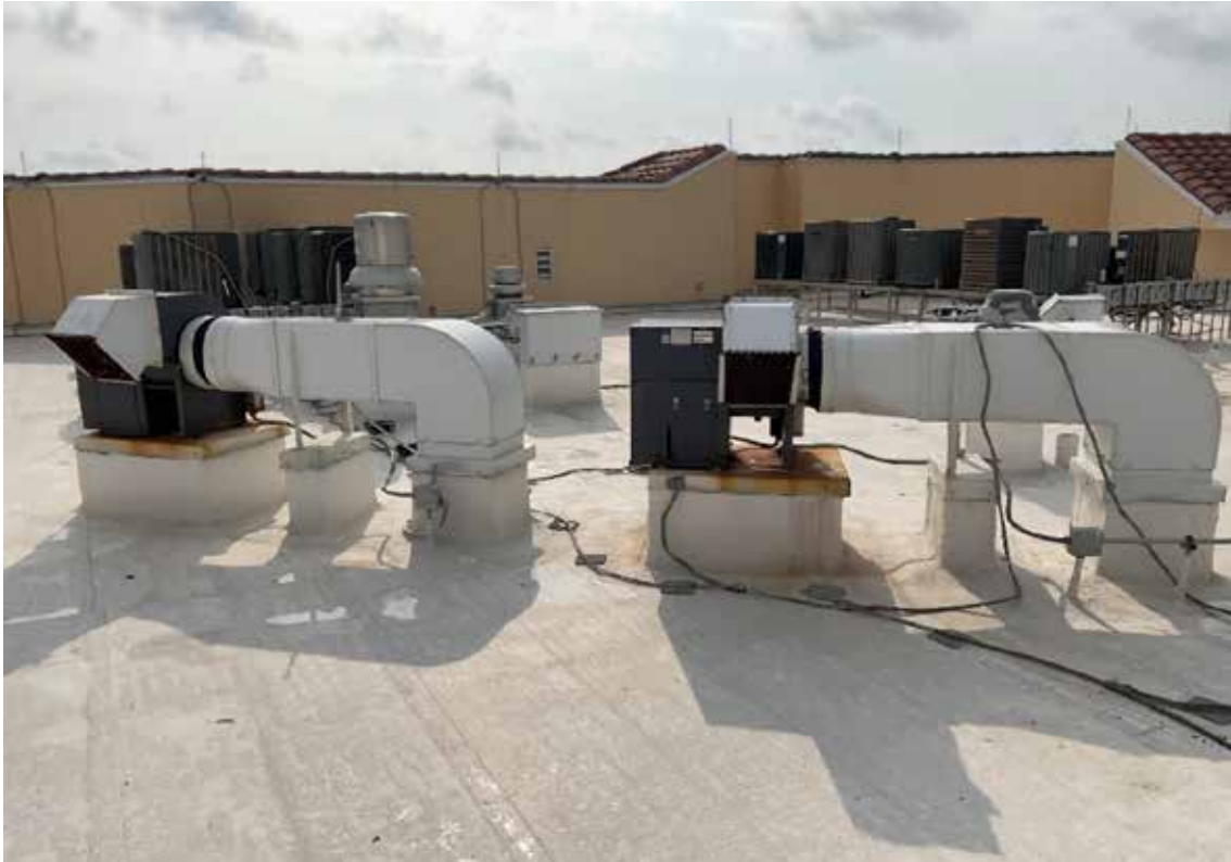
Roof Exhaust Fans
