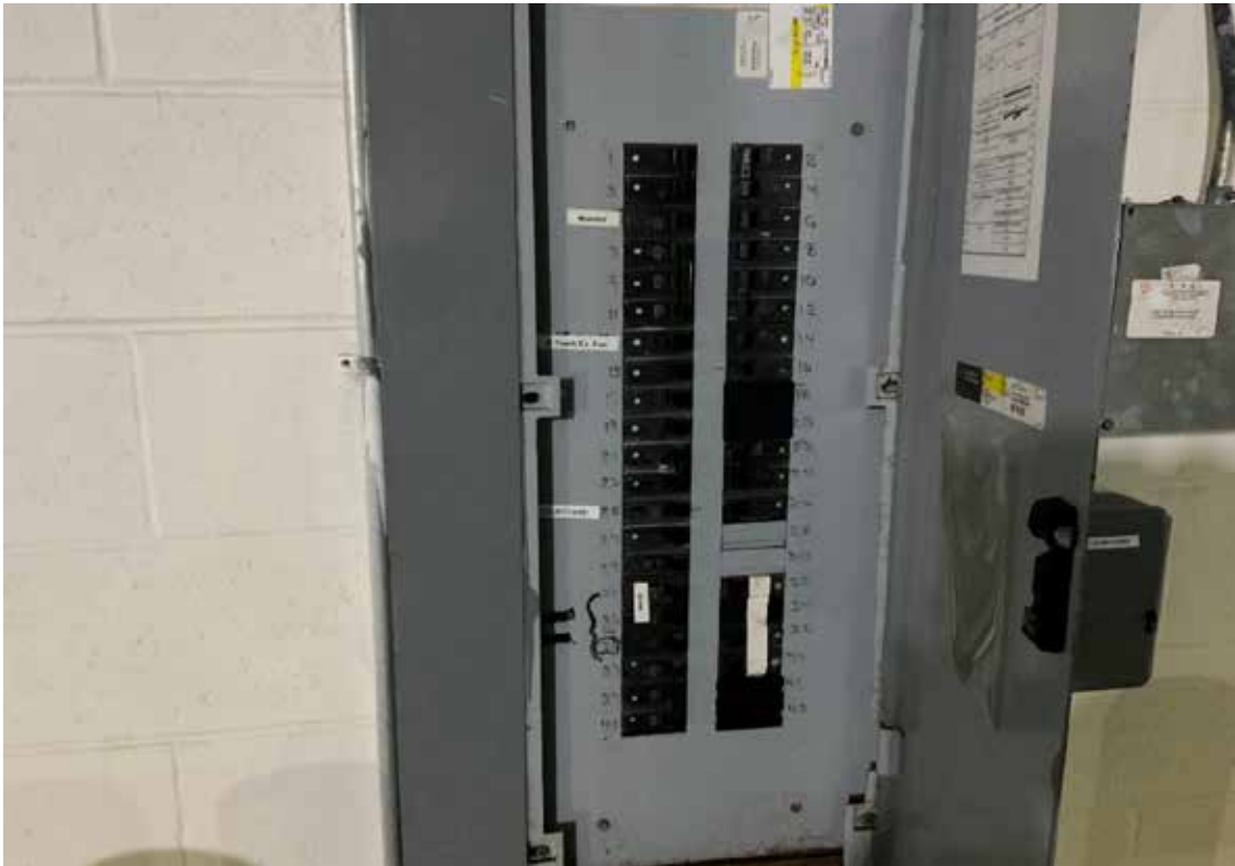
Electrical Panel 1HB
