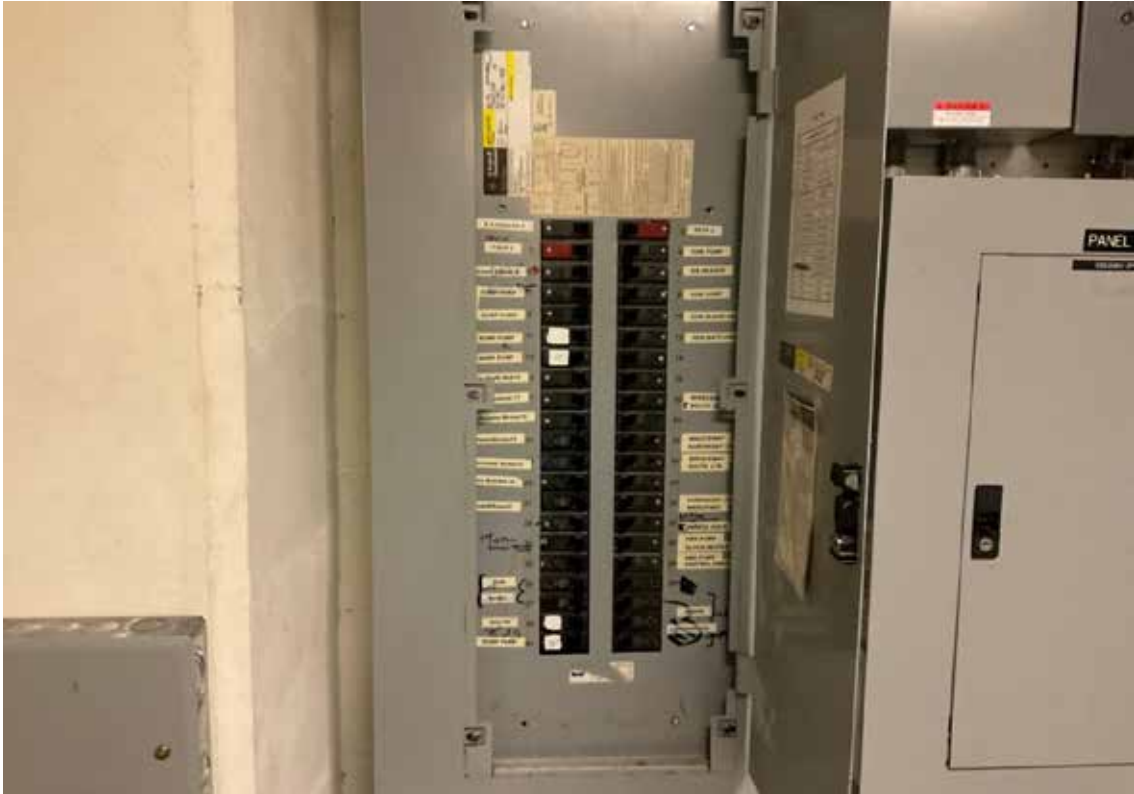
Electrical Panel 1EM
