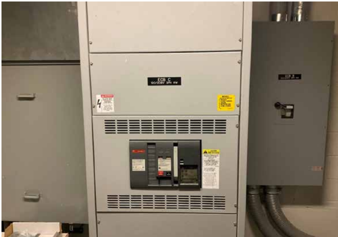
Electrical Panel ECBC
