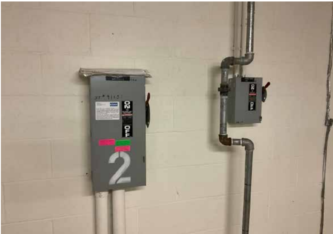
Elevator Control Shut Off
