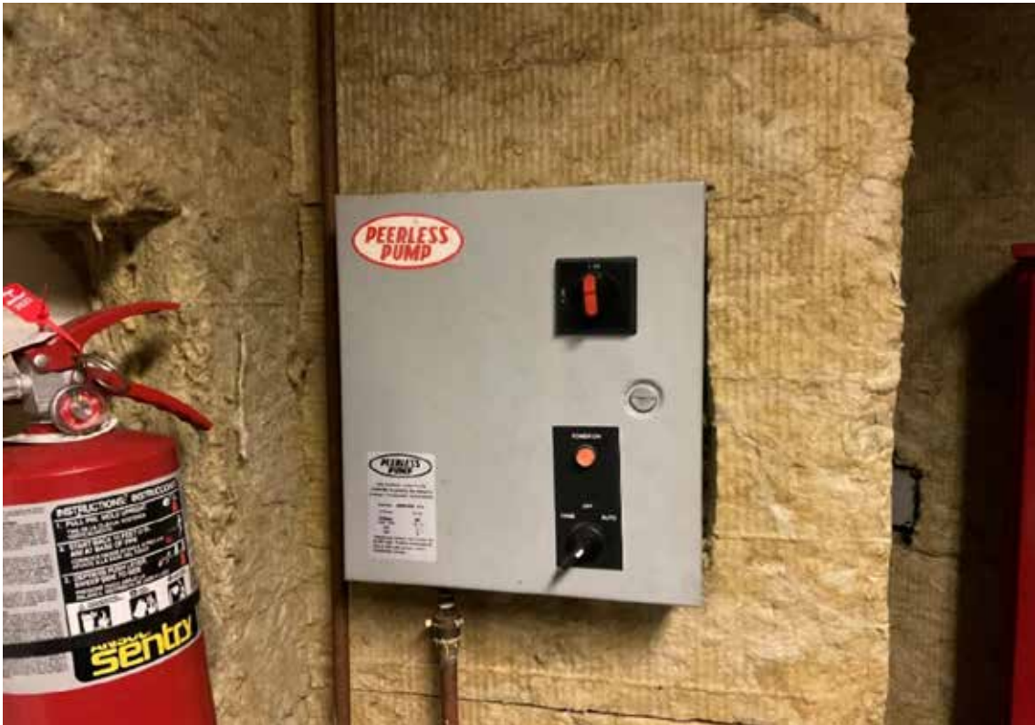
Fire Jockey Pump Controller
