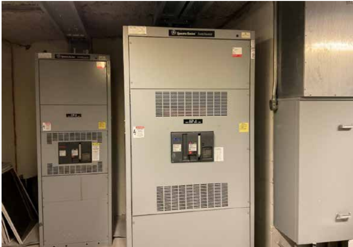
Electrical Panel ECBA
