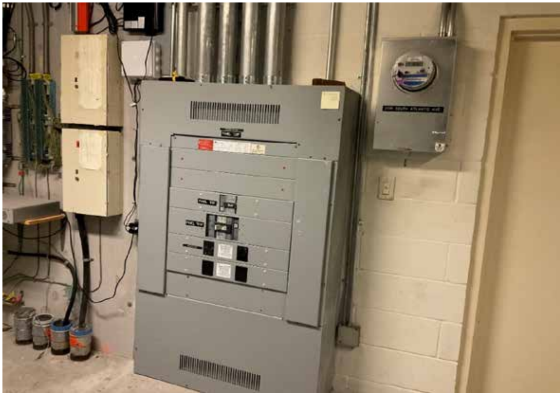
Electrical Panel EDP
