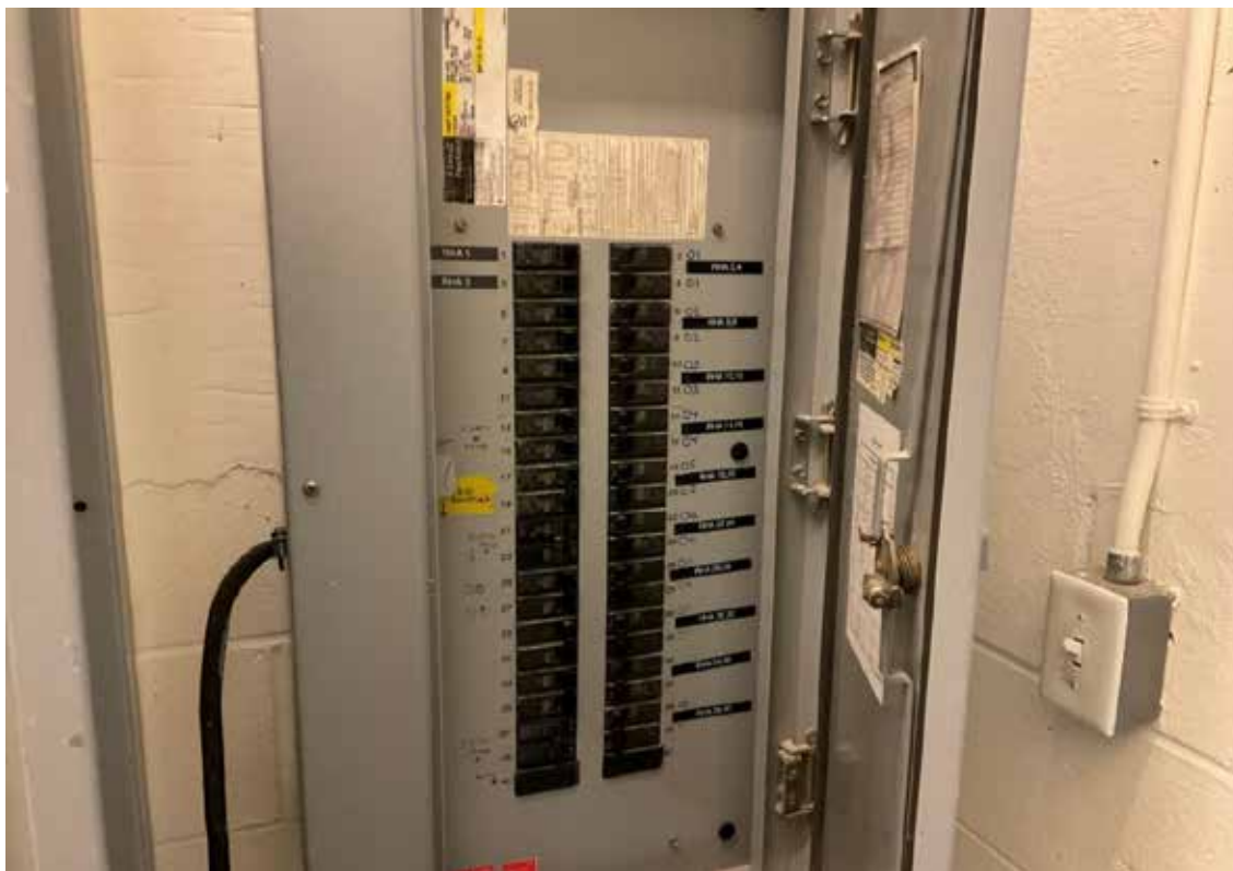
Electrical Panel RHA
