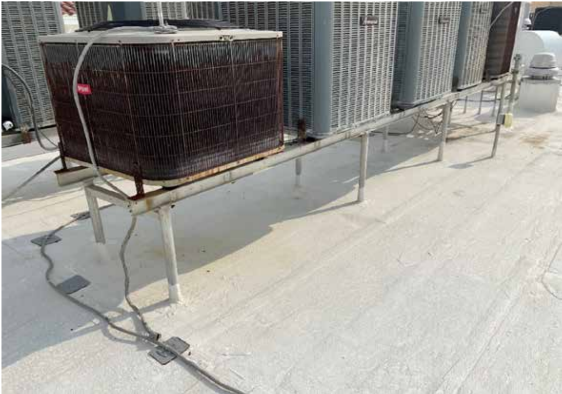
Roof A/C Stands
