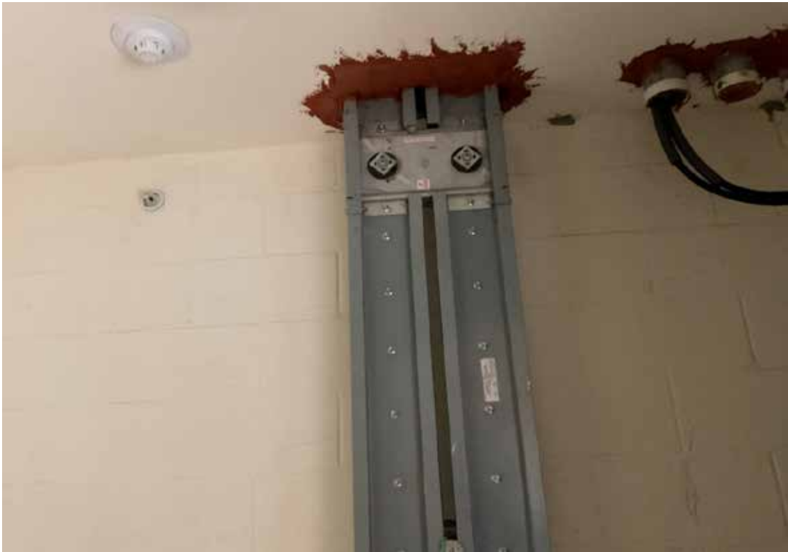
Electrical Bus Line - Typical
