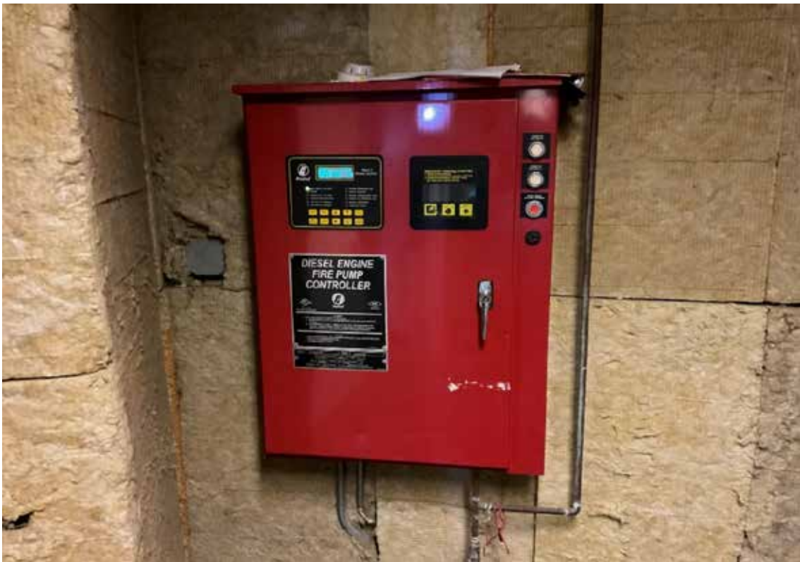
Fire Pump Controller
