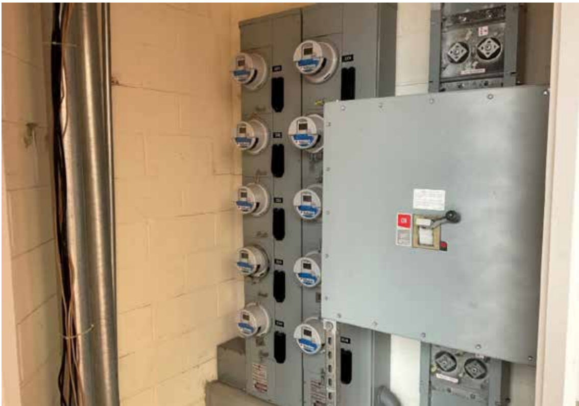
Electrical Meters - Typical
