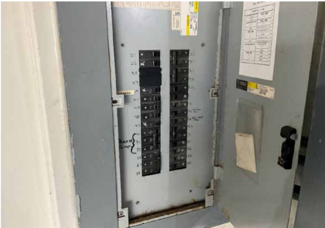
Electrical Panel 1HA
