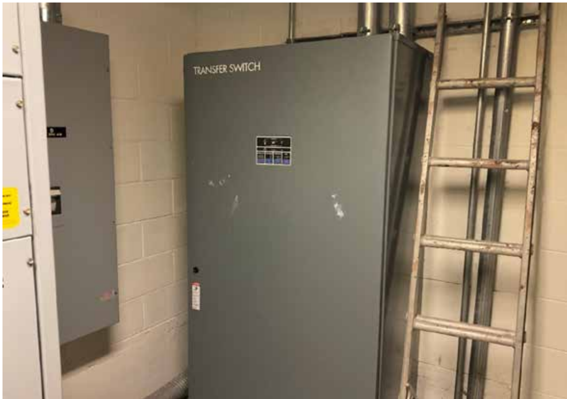
Generator Transfer Switch
