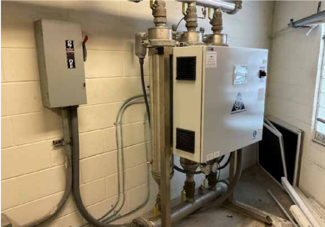
Domestic Water Pump System
